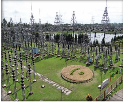
Chakmir Substation (CESC Ltd) – First Substation to be certified as “IGBC Platinum” in 2018
